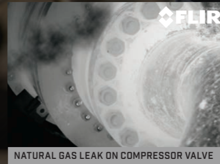
NATURAL GAS LEAK ON COMPRESSOR VALVE
