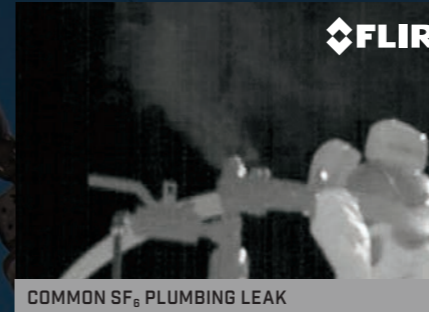
COMMON SF 6 PLUMBING LEAK
