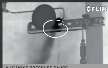
A LEAKING PRESSURE GAUGE
