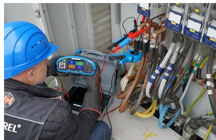
Iron Clamps connected to an external output to eliminate parallel resistances and current paths where several circuits are connected to live network.
