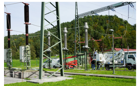
Measured result of live loop resistance on DC control circuits at the field end to be compared with battery source for evaluation of the conductors, relays and contacts quality.
